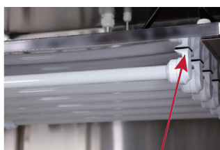
Lamp Holder Operational under High-Humidity Conditions
